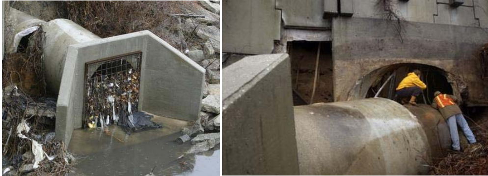
Figure 2. Images of storm drain culvert with debris accumulated behind grate, forcing the pipe to disconnect (left) and detached drain pipe from bridge structure (right). Photo credit: Muskegon Chronicle.
